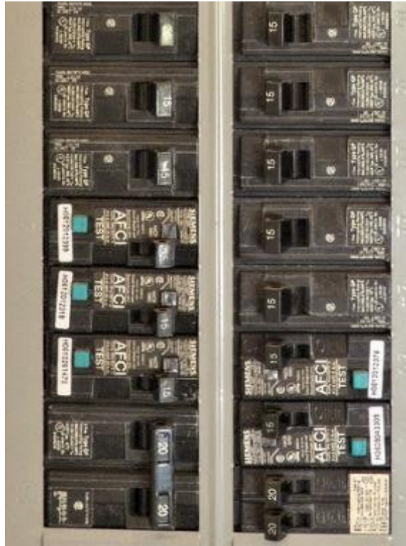
Figure 6. Breaker Box Equipped with GFI Breakers.
